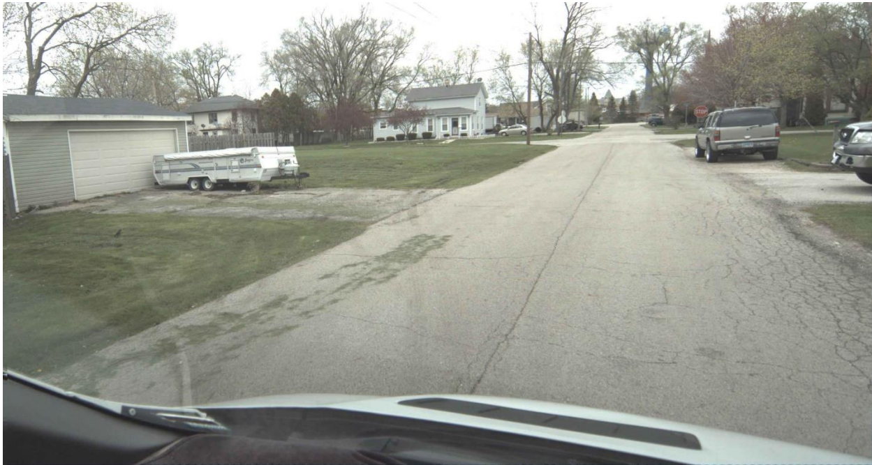
Figure 11 - Example of a Pavement (roadway) Rated as Poor
