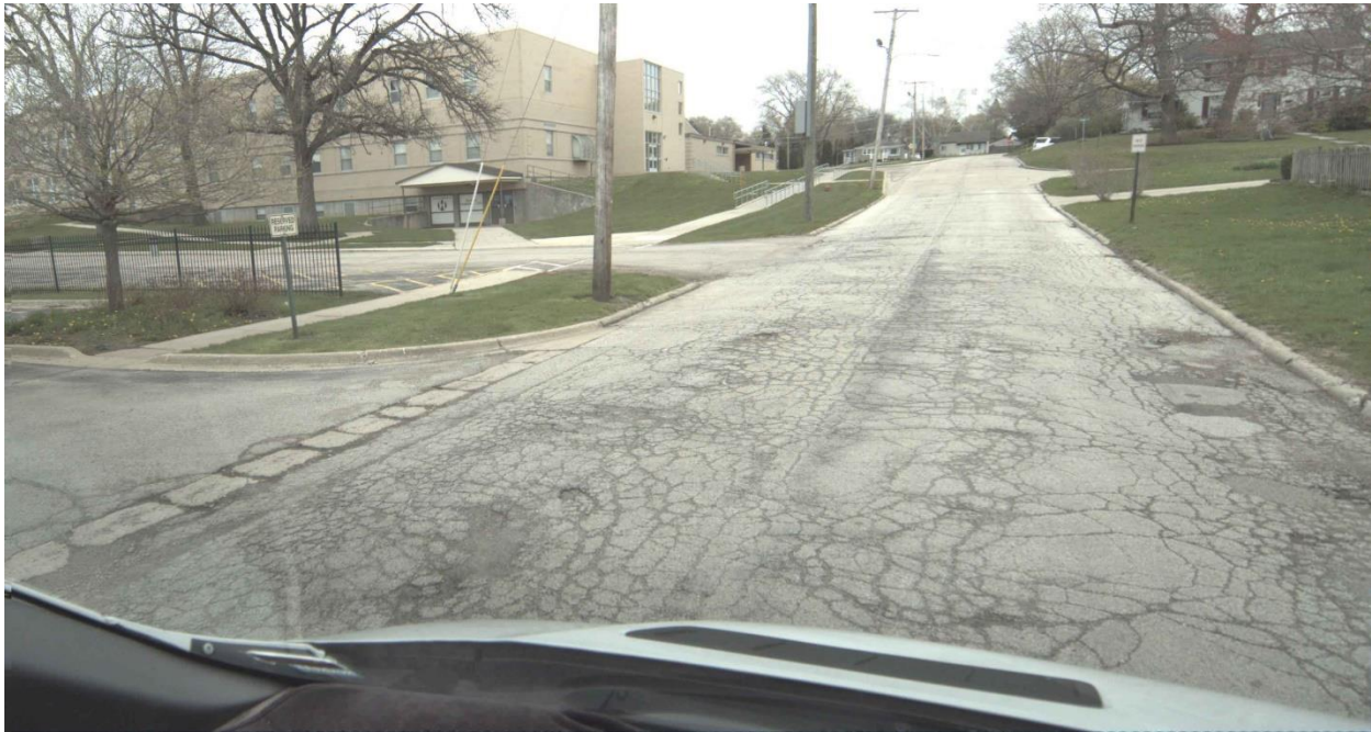
Figure 9 - Example of a Pavement Rated as Serious
