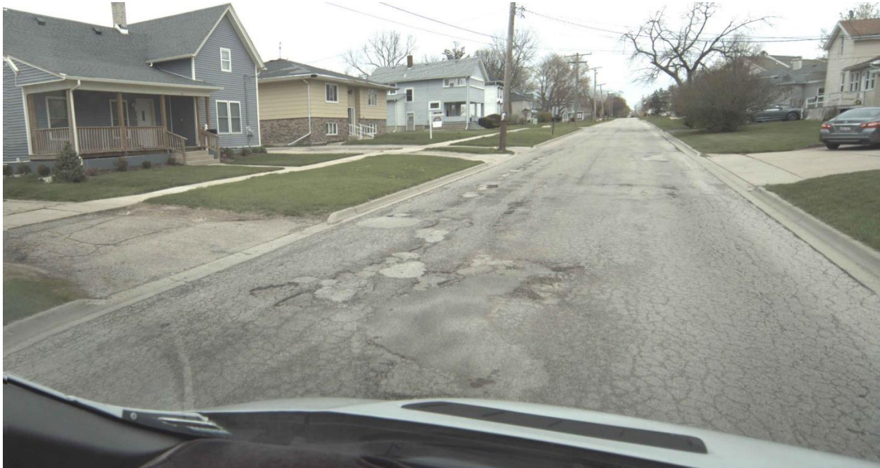
Figure 8 – Example of a Pavement Rated as Failed
