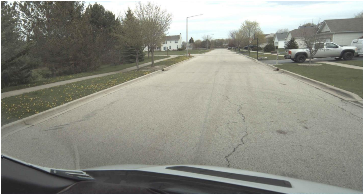
Figure 12 - Example of a Pavement Rated as Fair
